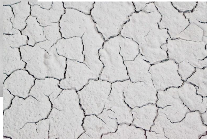
Fig 4. Cracked paint as a result of too much paint being applied. (Right)
