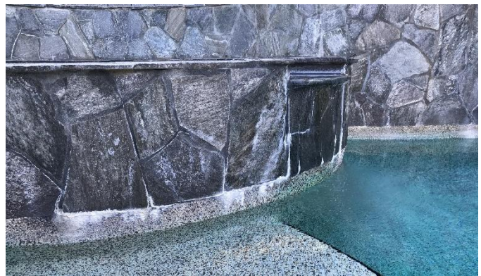
PHOTO: Efflorescence looks like carbonate scale because it is also calcium carbonate (CaCO 3 ). But it is from moisture pushing through the concrete wall of the raised spa, taking minerals with it to the outside.
