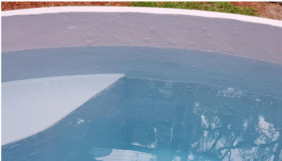
General view inside the plunge pool showing blisters above and below the water line.
