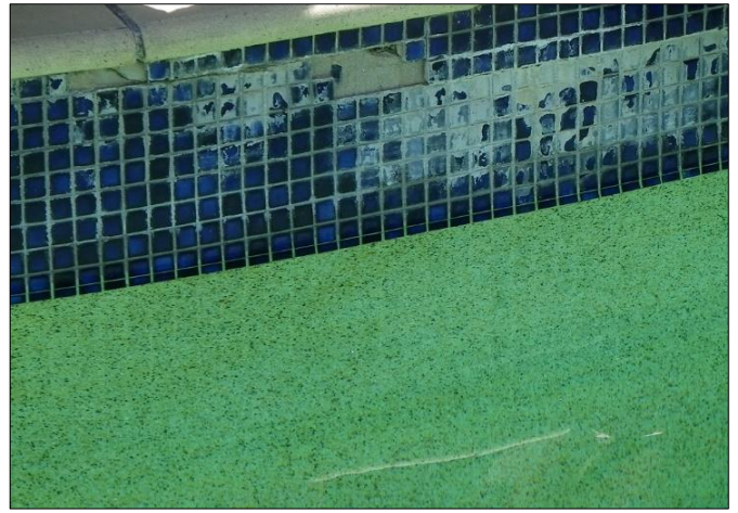
Figure 4 So many water related issues resulting in tiles being pushed off. Note area below tiles seems fine, as being porous.
