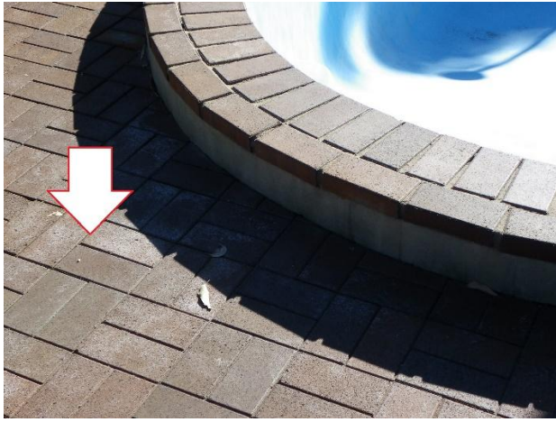
Figure 3 Dark pavers and coping with efflorescence present, with drainage. Resulted in blisters on pool walls.
