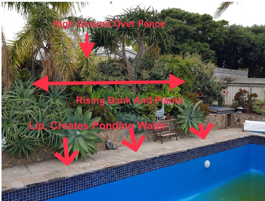
Image 2 Here is a pool with rising ground along one side (rises higher on neighbour's land) and combined with the rising bank and garden, is a great trap for rainwater and resultant seepage. (Into or under pool)
