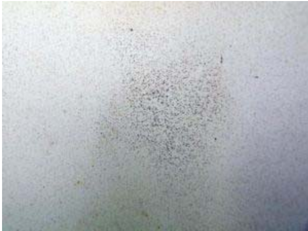
(Photo 2) – Pinpoint rusting through the topcoat. Cracking/Brittleness of Coating
