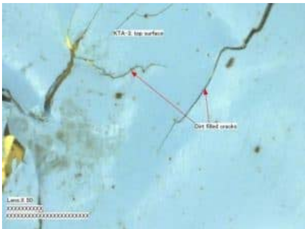
(Photo 3) – Cracked topcoat of a system applied approximately 20 mils below the minimum specified thickness range.
