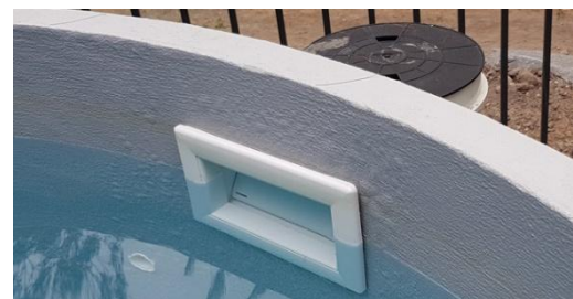
Fig 4: (right) Blisters forming in pool paint due to the leakages in #3 and the effects of “wicking” and hydrostatic pressure.
