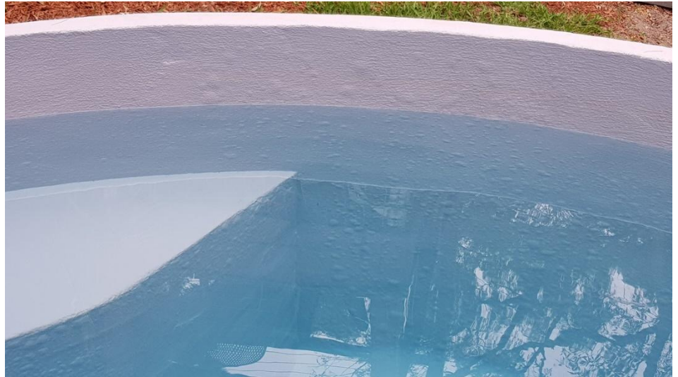
Fig 6: General view inside the plunge pool showing blisters above and below the water line. See discussion below for reasons why and how to prevent it happening.
