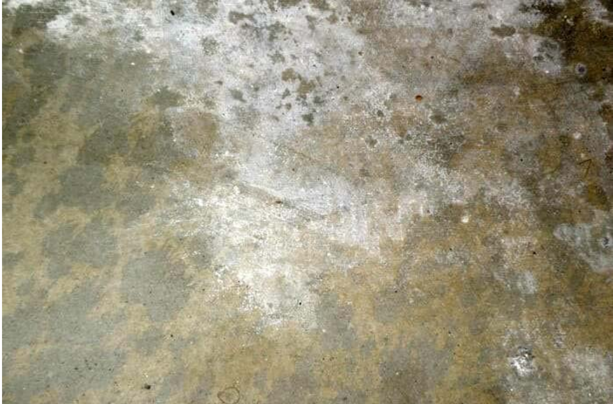
Efflorescence caused by moisture in the concrete
