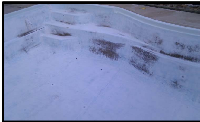
Worn gel coat in fibreglass pool. Needing attention.
