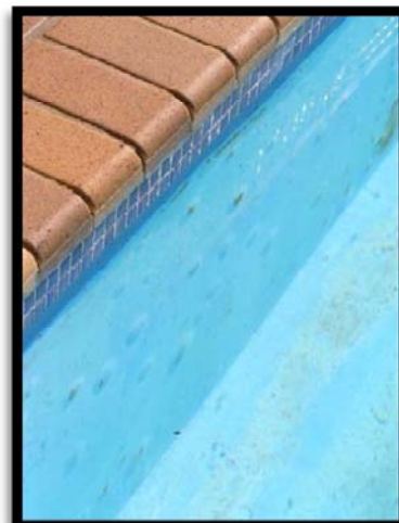
Osmosis on wall of fibreglass pool
