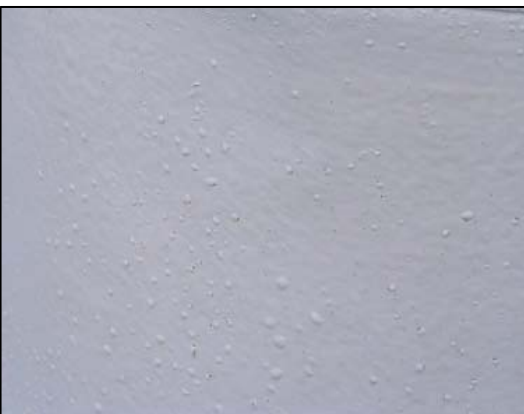
Figure 5 Painted wall showing hydrostatic blisters
