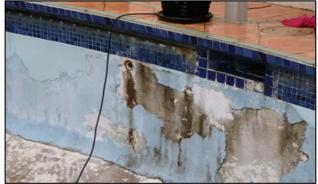
Figure 4 Effects of poor drainage around pool and causing in part delamination of render.
