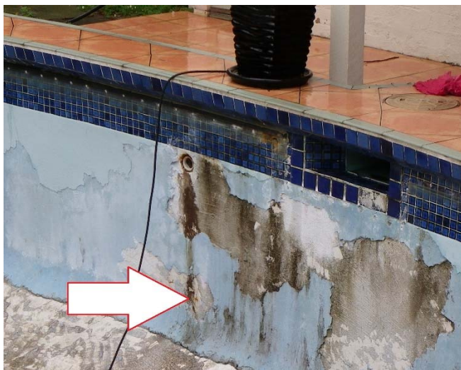
Figure 7 Extensive issues due to water trapped behind wall.
