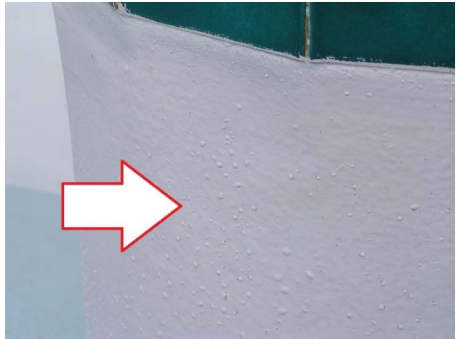
Figure 6 Hydrostatic blisters in painted surface, due to water (leakage, building up) behind pool shell.
