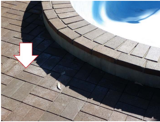
Figure 3 Dark pavers and coping with efflorescence present, with drainage. Resulted in blisters on pool walls.
