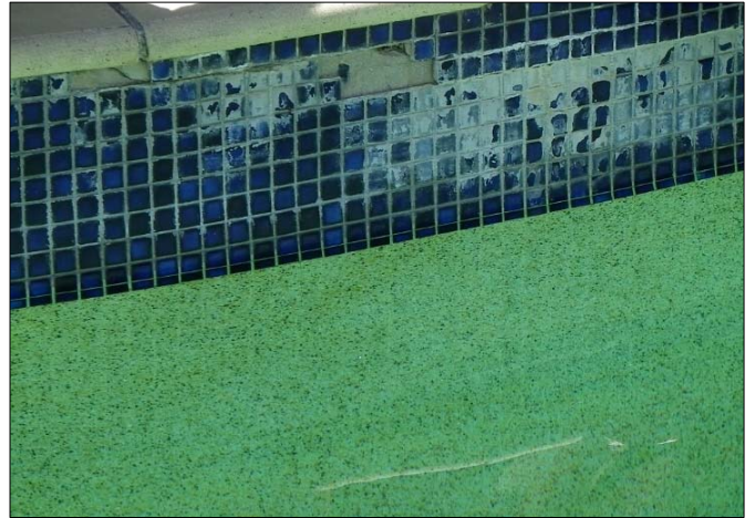
Figure 4 So many water related issues resulting in tiles being pushed off. Note area below tiles seems fine, as being porous.
