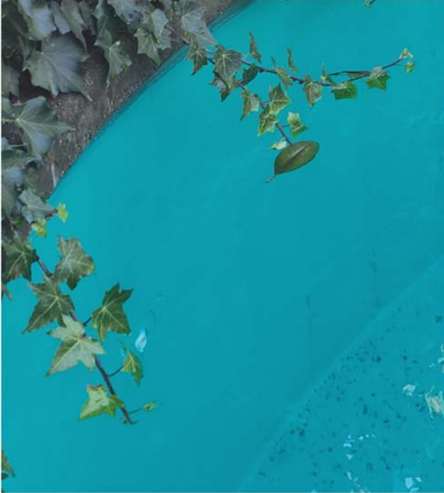
Over hanging Ivy creating algae on pool floor.
