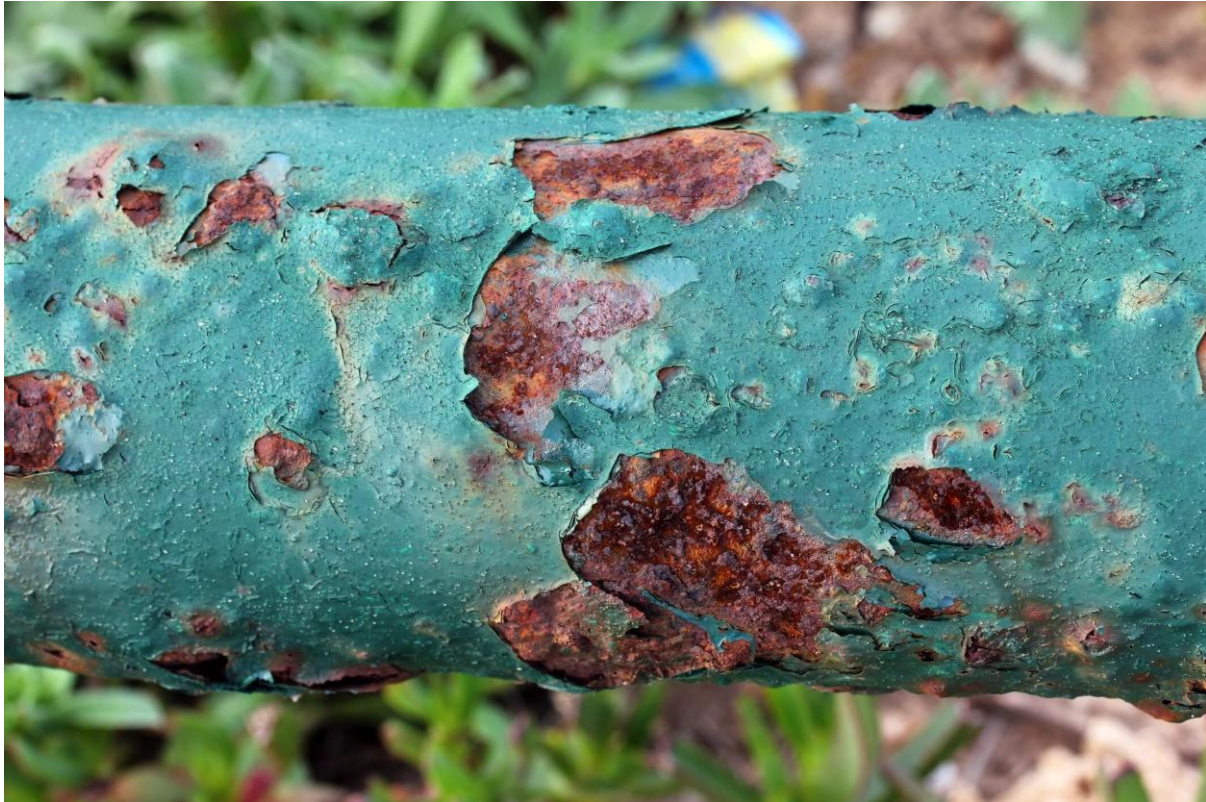
Figure 4. Undercutting caused by corrosion products forming on a metal pipe (Felix Bensman / Dreamstime.com).
